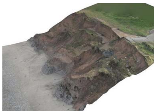
Fig. 13 Orthophoto image of coastal cliff landslide produced using UAV photogrammetry, Aldbrough, UK (2013), BGS©UKRI[2018]
