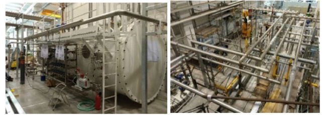
Figure 11. View of the on-going assembly of MITICA cryogenic plant—auxiliary cold box (left) and piping layout inside the building for auxiliaries (right).
