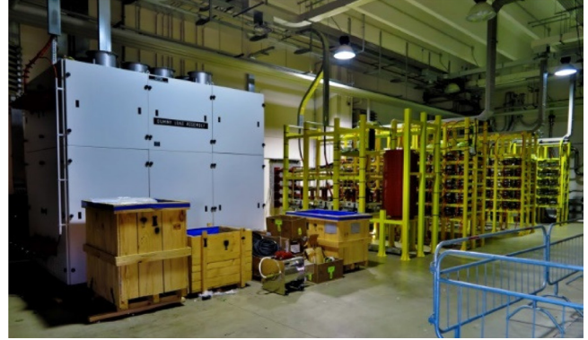
Figure 1. SPIDER accelerator power supplies: left, dummy load; right, insulating frames with pulse step modulator modules.
