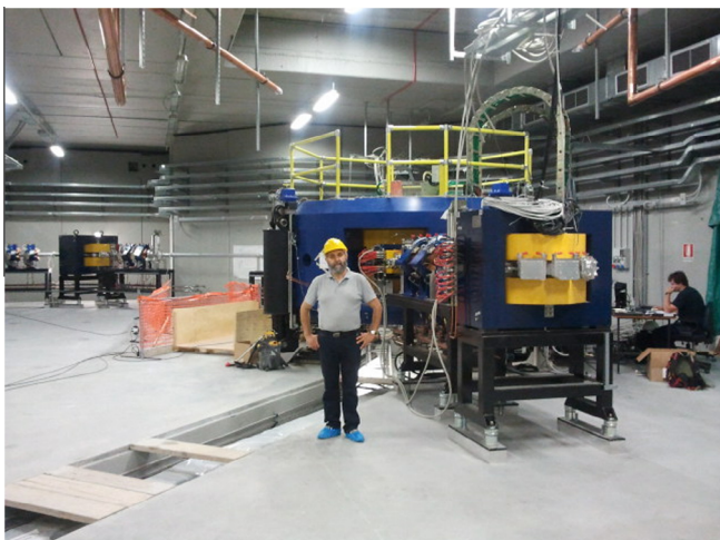
Fig. 3. Photo of the SPES cyclotron and beam line during installation.
